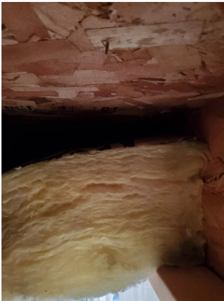
Classic case of fiberglass gone wrong. Does not completely fill cavity and no air sealing along perimeter.
